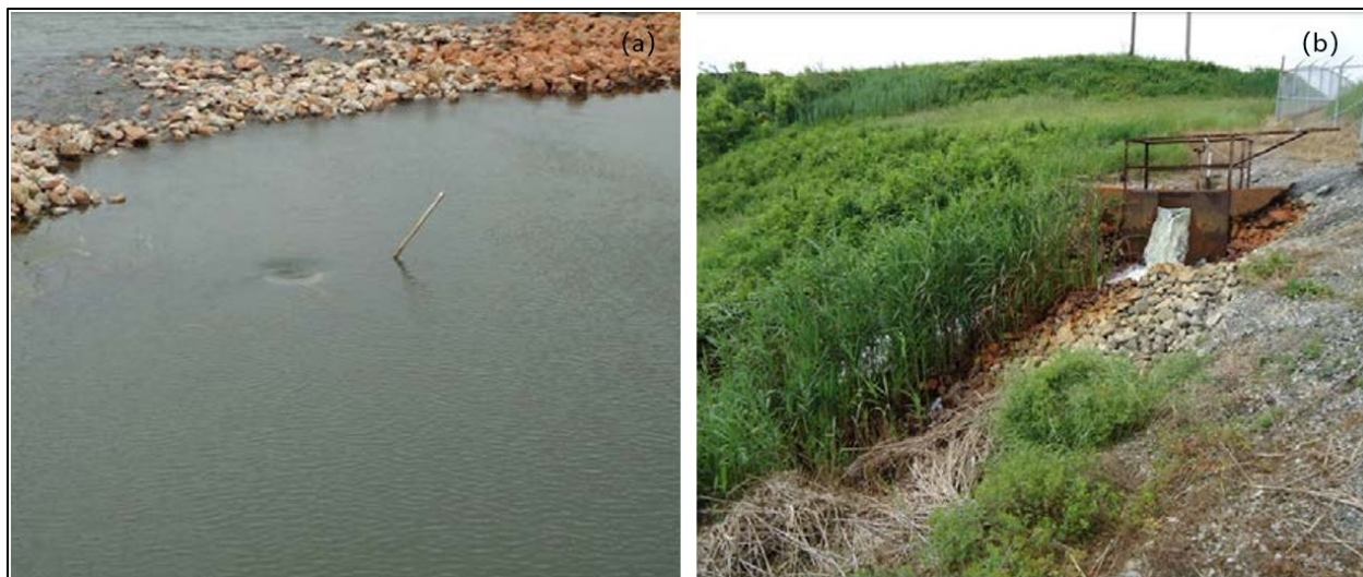
Figure 3.4 2011 Photographs of Pond 4 – (a) Intake from Pond 4 to Outlet Structure (pipe submerged); (b) Outlet Structure from Pond 4. Source: Kleinfelder, 2013.
